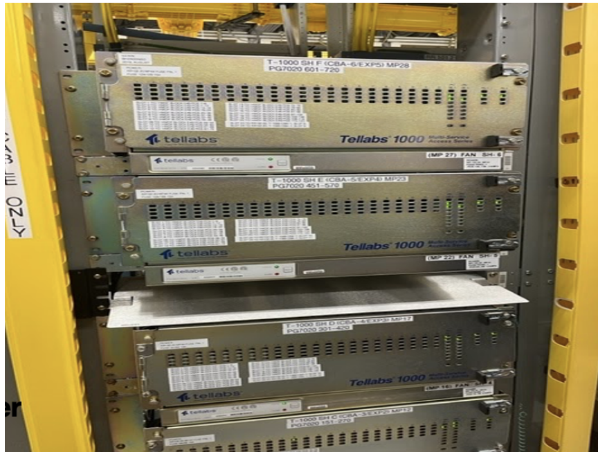
Figure 5-3: Picture taken showing individual T1000 fiber-based switch which can handle similar traffic as TDM switches, using a fraction of space and energy.
