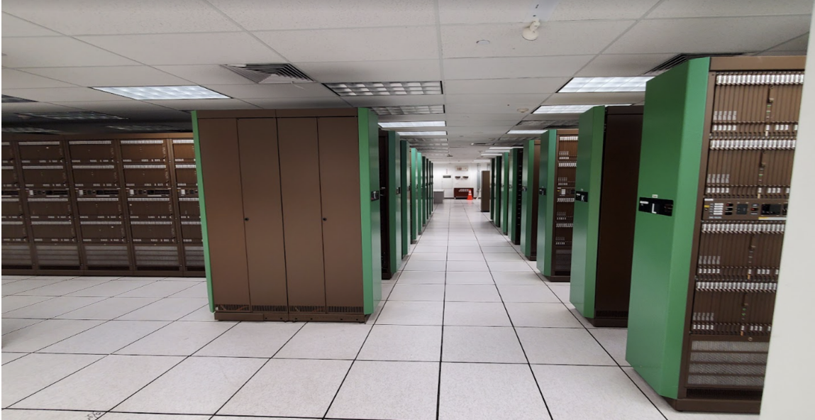
Figure 5-2: Picture taken showing floor of central office filled with rows of legacy TDM switches which still handle much of the copper network traffic.
